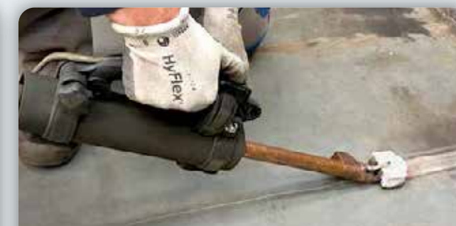
SHIPYARD - CONSTRUCTION NAVALE Inductor L20/B4 Powerduction 220LG
